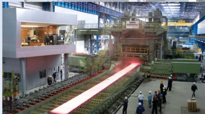
The analog addressable fire alarm and extinguishing system and intrusion alarm system for Stan 5000 of Magnitogorsk Metallurgical Combine, one of the largest Russia plants equipped with a state-of-the-art sheet-rolling shop
